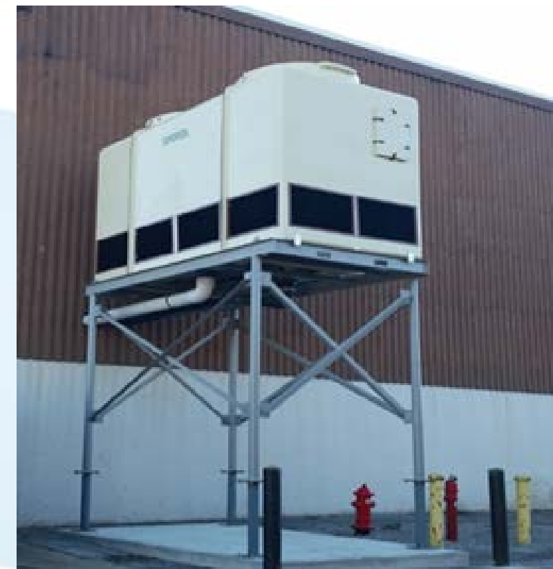
Cooling tower at Fort Wayne, Indiana, United States
